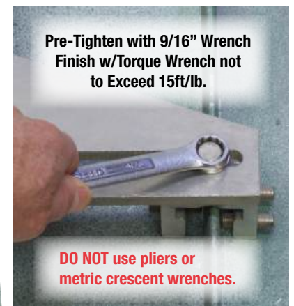
Fig.21 Base Plate Bolts
